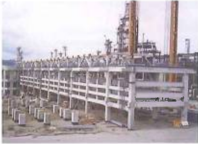
Esperaldas Pipe Rack, Ecuador
